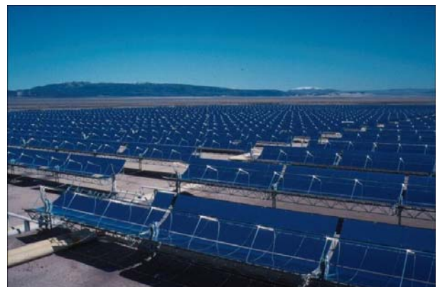
Parabolic trough collector field for the CSP power plants in Kramer Junction, California
